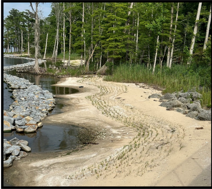
A granite sill installed to reduce wave energies and prevent future erosion was constructed on MCAS Cherry Point's shoreline. Over 130,000 native marsh grasses were planted to stabilize the site and restore the ecosystem.
