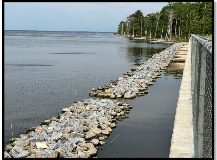
Sediment is seen accumulating behind the granite sill almost immediately after construction. Over time, this shoreline protection will restore government lands that were lost to erosion.
