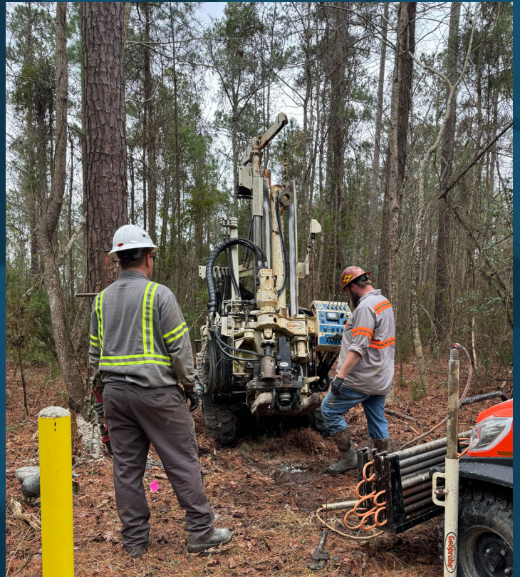
EC/HPT probes were advanced using direct push technology drilling techniques to collect continuous data on formation permeability and lithology.
