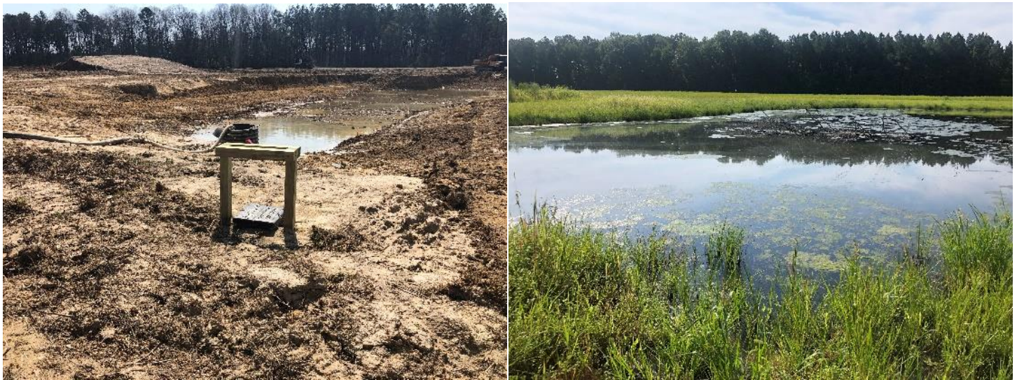
The before (left) and after (right) of the 5-acre wetland restoration project at Cedar Point Wildlife Management Area in Welcome, Maryland.
