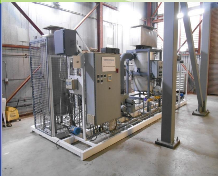
iSCWO Test System at General Atomics
