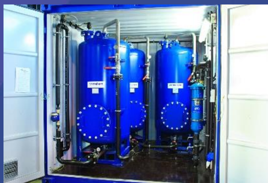
Figure 1. (Top) Mobile PFAS Removal System Schematic. (Middle & Bottom) German Mobile Treatment System.
