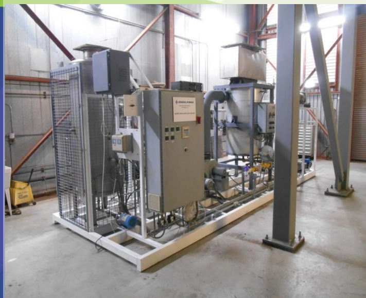
iSCWO Test System at General Atomics
