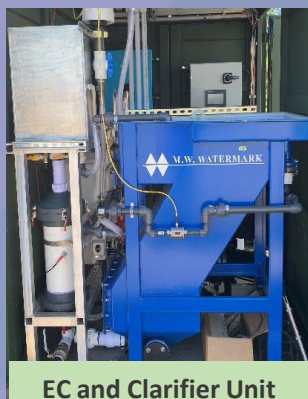
EC and Clarifier Unit
