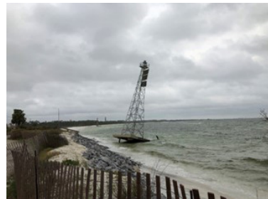
Shoreline damage along NAS Pensacola following a storm. Credit: Escambia County NRM.
