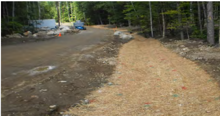
Road and drainage repairs at GPOAC. GPOAC is located within the Atlantic salmon watershed.
