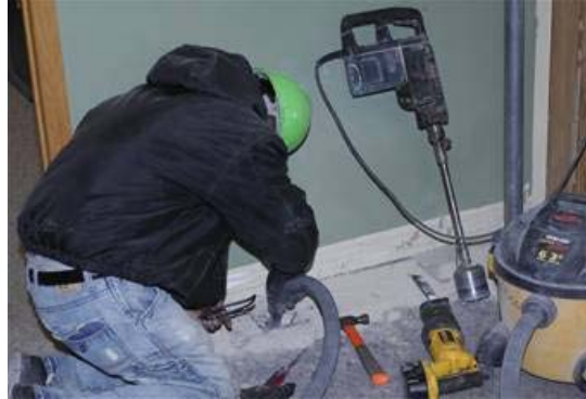
MINOT AIR FORCE BASE, N.D. -- A construction worker drills a hole through a floor in the 5th Bomb Wing headquarters building here Dec. 15, while installing a geothermal heat system. The 5th Bomb Wing headquarters building is currently undergoing construction to utilize geothermal heating by having 39 ground source heat pumps installed in the building along with 30 geothermal wells on the west side of the building. (U.S. Air Force photo by Staff Sgt. Keith Ballard)
